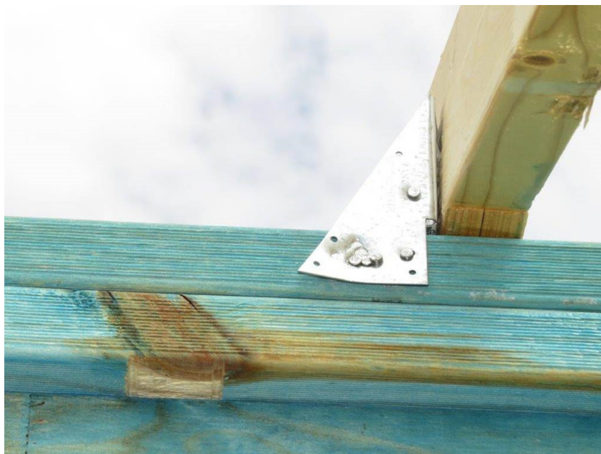
Photo 1: - Example of framing anchor not correctly nailed off and fixed to ribbon plate only
